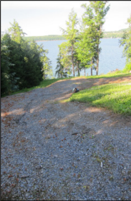
Improper crowning and siting of this camp road led to nearly immediate erosion and deposition into the lake after significant tree removal.
