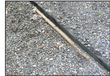
Water deflectors are installed so that 3" of the rubber belting extends above the surface of the road.
